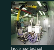
Inside new test cell
